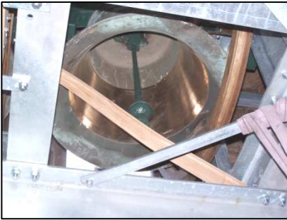
Re-tuned bell & bell frame
